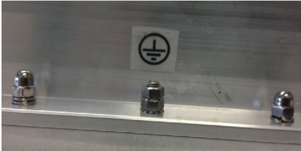
Figure 44: 9502 Protective earth grounding
