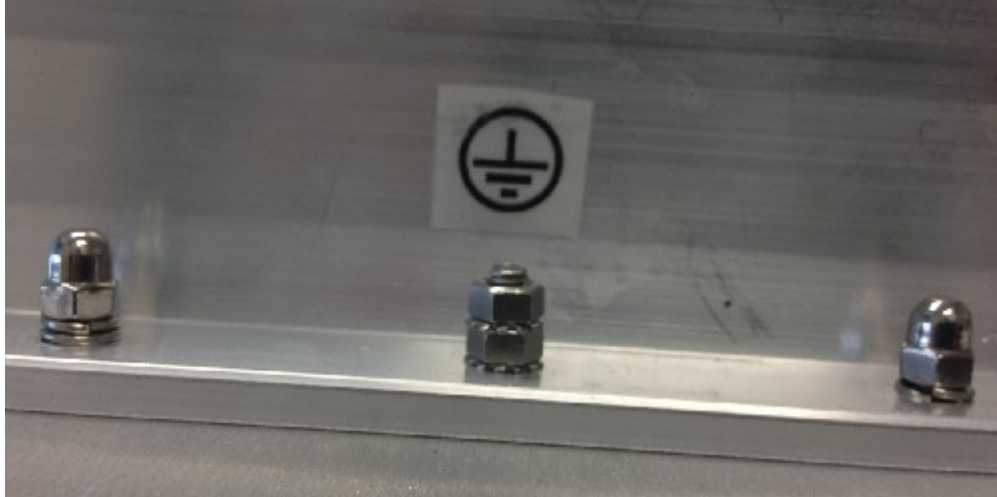
Figure 48: 9502 Protective earth grounding
